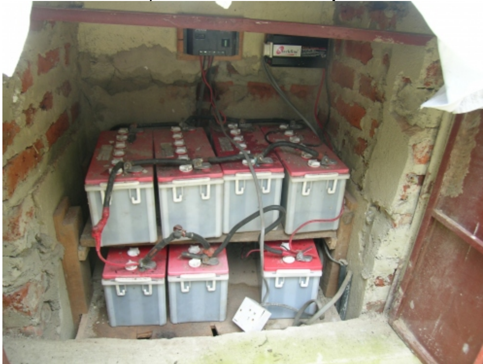
Tourist lodge lighting system
